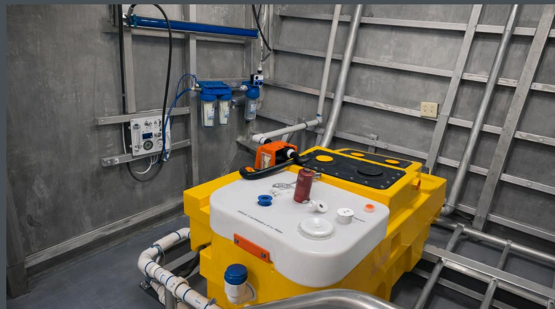
WATER MAKER & SEWERAGE PLANT
